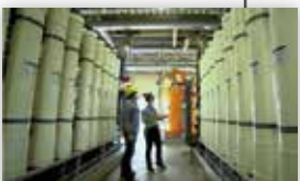
Seawater Desalination: 28,000m 3 /d
