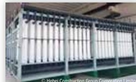
Wastewater Treatment: 315,000m 3 /d
